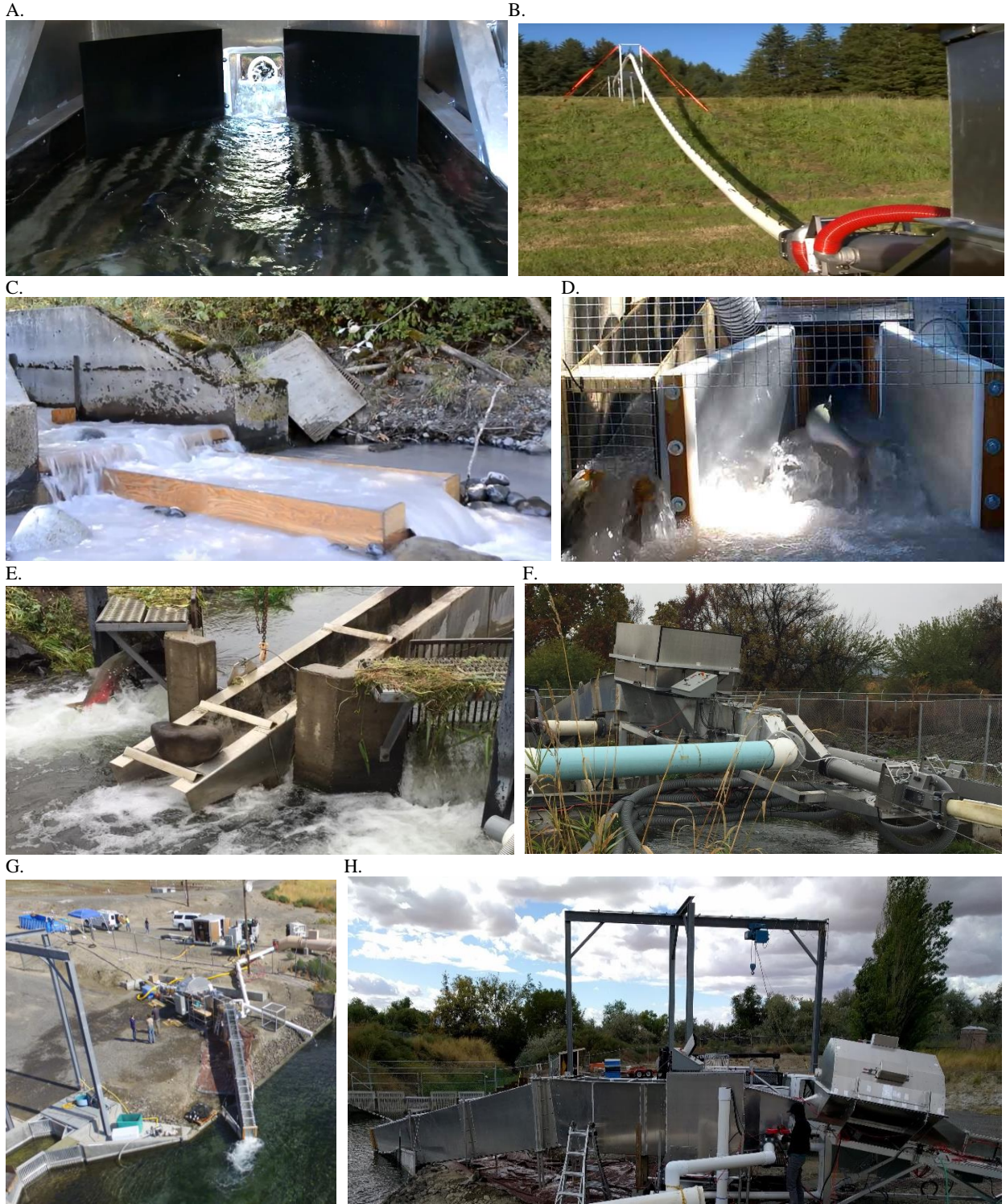
Figure 6. A&B City of Newport, OR water flow attracted Rainbow trout for volitional entry with false weir just above the surface level. C&D White river pool and weir steps providing pink salmon with false weir access for volitional WFTS entry. E&F Prosser hatchery steeppass in a stream of the Yakima river combined with a study WFTS with the prototype scanning sorting component. Chinook and Coho volitionally entered WFTS. G&H Ringold Springs Alaskan steeppass and flow box facilitated volitional WFTS entry of Columbia river Chinook and steelhead.
